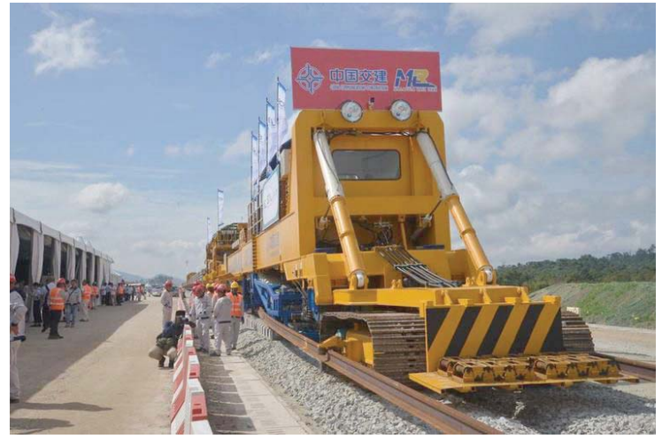
This photo shows the launching site of the East Coast Rail Link project in Kuantan, Malaysia, on Dec. 11, 2023. (Photo by Xu Xinyu/Xinhua)
